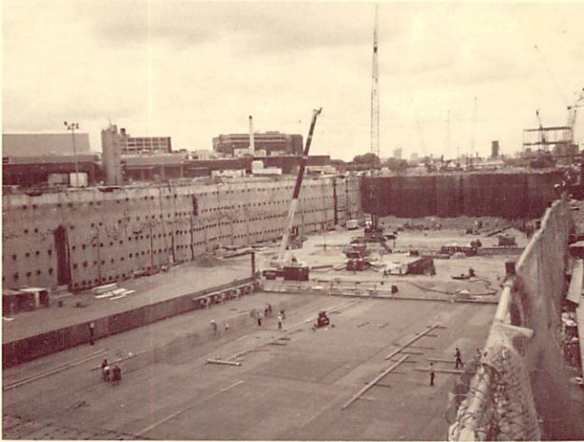
The casting basin for the construction of Modern Continental's sunken concrete tubes.
