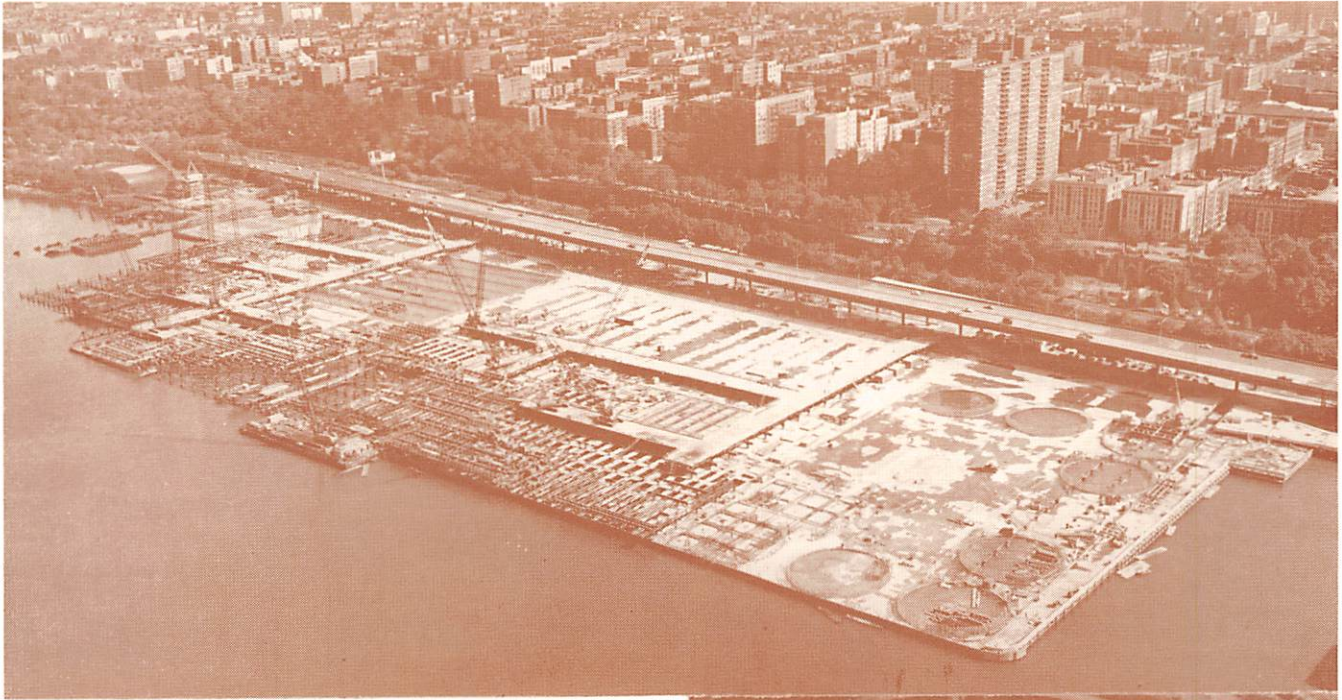
Perine North River Associates — Charles Edgar, Project Manager. 28 Acres of Sub Structure on 2300-42" Caissons for North River Water Pollution Control Project.
