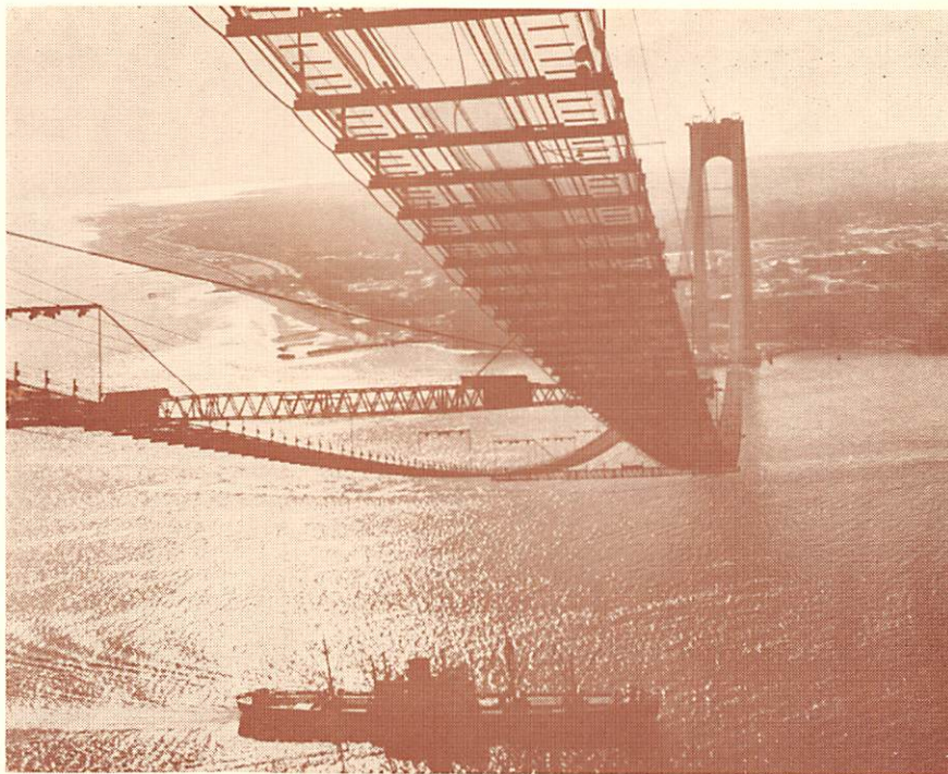
NEW NOTE in New York's skyline symphony: the 20-foot-wide catwalks slung between the towers of the Verrazano-Narrows Bridge, world's longest suspension span. This is one of the sites — and sights — to be visited by our Students' Day tours on April 26. This view looks toward Staten Island, from the Brooklyn side.
